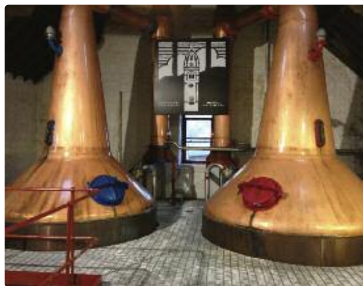
Wash and spirit stills and copper condensers.
